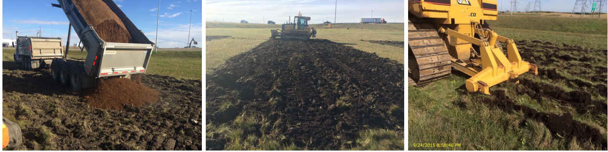
Figure 2. The tracked piece of equipment used to spread organic amendment evenly on the Pulp and Paper Residuals and Compost planting beds (left). Right: three rear-mounted tines (60 cm depth) were also used on all three trial sites to perform deep ripping. This was performed on all treatment beds except the 'control' beds.
